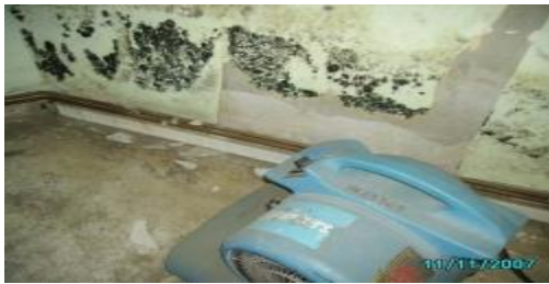
Dirty fan spreading mould and surface contamination
